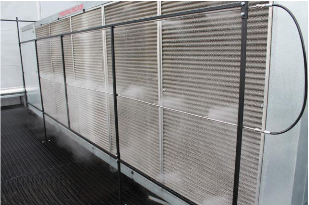
Adiabatic cooling of a chiller with Ditusz high pressure mist-cooling
